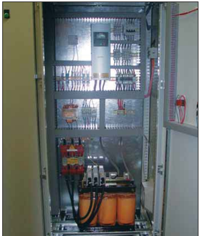
Interno quadro "VARIAS" "VARIAS" inner of electric panel
